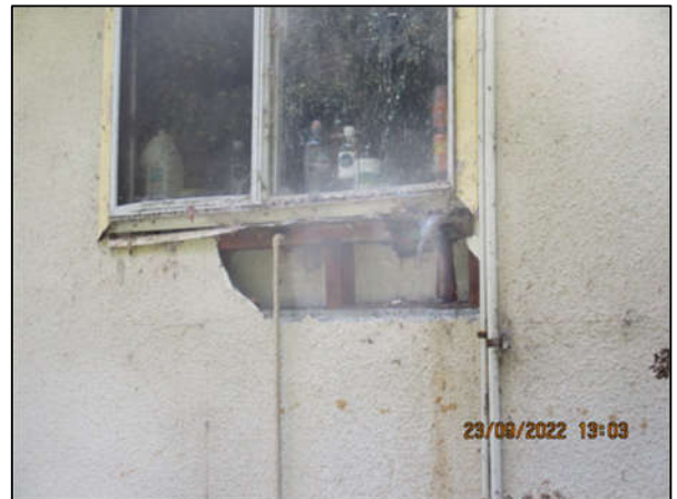
External cladding damage
